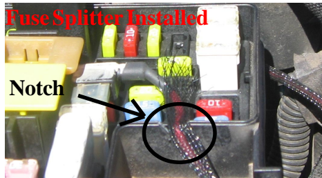
Figure 3: JK Power Connection
